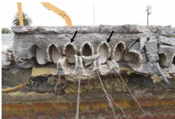
Fig. 2: Fractured concrete roof panel. BSA-caused deterioration manifested as paste color lightening and weakening along the cell perimeter (arrows) as well as corroded and broken prestressing strands
