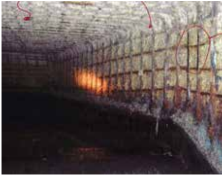
Fig. 7: Sewer tunnel with exposed second mat of steel reinforcement. Top concrete and the first mat of steel reinforcement were reportedly lost to the existing surface (from Reference 7)
