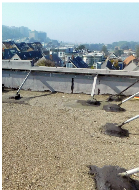
FIGURE 1. PARAPET BRACING OF AN UNREINFORCED MASONRY PARAPET IN A HIGH SEISMIC REGION
