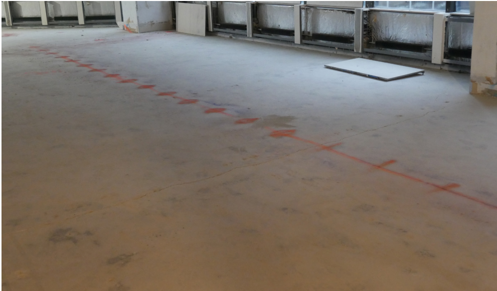
Figure 3. Marked locations where headed shear connectors are to be installed, spaced along steel beam below and identified using GPR.
