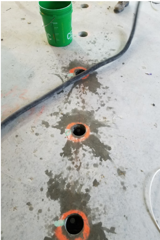
Figure 4. Core holes in concrete slab spaced along span of steel beam below.
