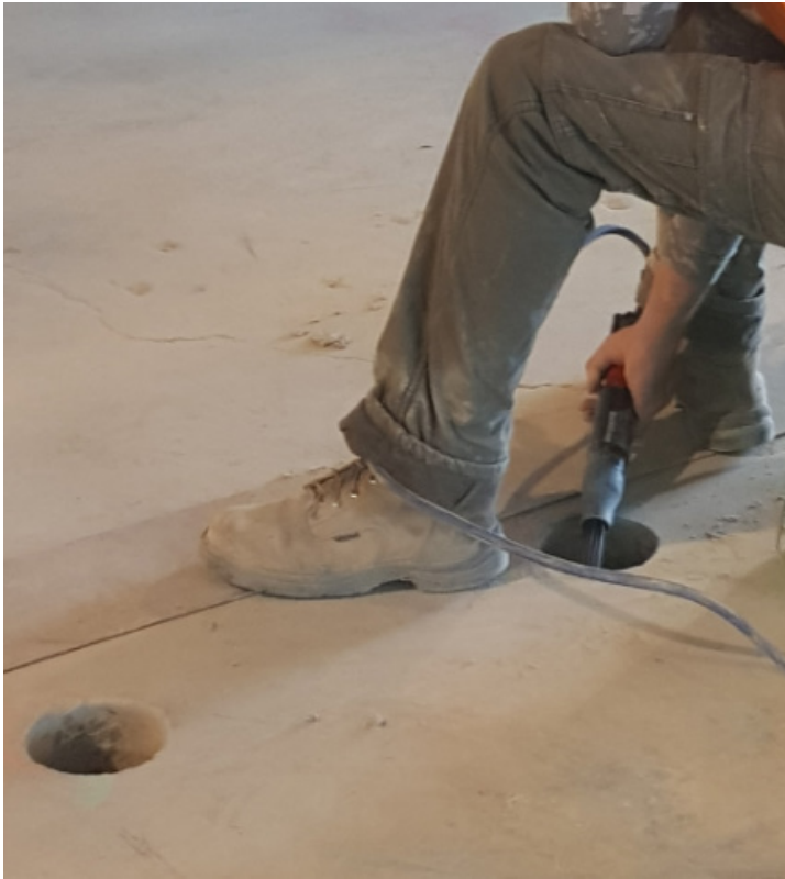
Figure 5. Mechanical abrasion at core holes.
