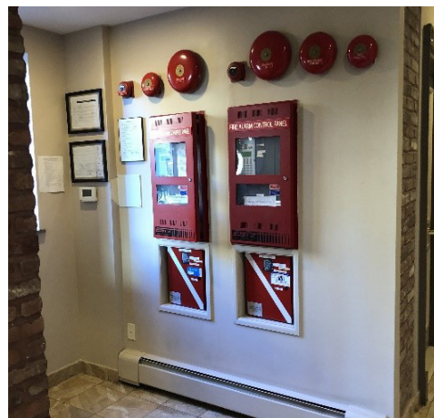
FIRE ALARM SYSTEMS CAN BE COMPLEX, SUCH AS THIS BUILDING THAT IS PROTECTED BY TWO INTERCONNECTED SYSTEMS.
