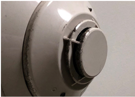
VISUAL INSPECTIONS CAN REVEAL DEFERRED MAINTENANCE SUCH AS THIS SMOKE DETECTOR WITH SIGNIFICANT PARTICULATE ACCUMULATION.
