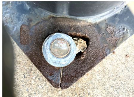
Figure 7. Oversized bolt hole.
