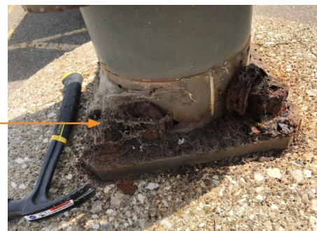
Figure 6. Same pole from Figure 5, with base plate cover removed, revealing corrosion and debris.
