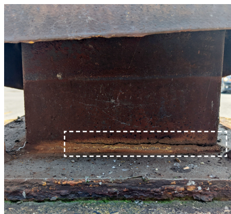
Figure 10. Crack at welded connection to base plate of square pole.
