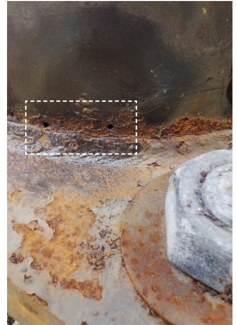
Figure 14. Holes punctured in subject pole by light tapping with hammer.
