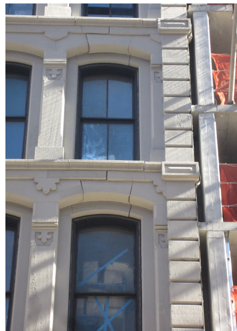
Figure 1. Cracking and displacement of existing stone arches due to foundation settlement associated with adjacent construction. New floor slabs also extend into a required seismic gap, where they can apply damaging earthquake loads to the existing building.
