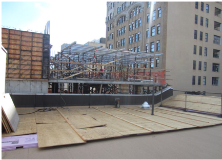
Figure 2. Inadequately secured sheets of plywood, intended for roof protection, can be dislodged by wind. This city's building code requires the plywood to be fastened over a layer of scaffold plank.
