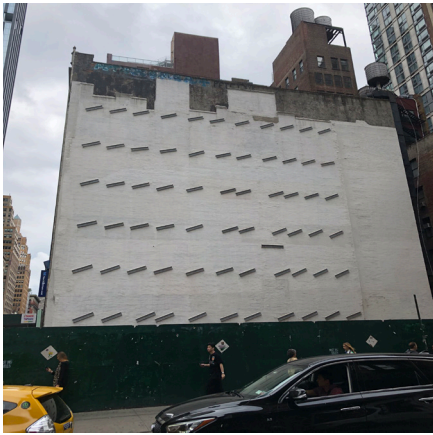
Figure 6. Former shared wall following demolition of existing building, with short lengths of steel channel attached to anchors bracing the masonry to floor structure at each level.
