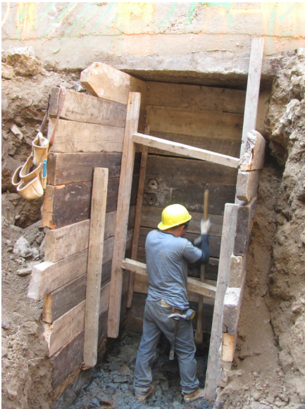
Figure 4. Timber sheeting at underpinning approach pit with adjacent areas improperly excavated alongside the existing foundation, increasing the risk of soil movement.
