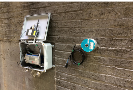
Figure 3. Installation of seismograph (at right) and monitoring data logger (at left) in progress at foundation wall of existing building.
