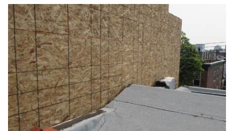
Figure 5. This interface between a rising wall and an existing roof will require careful detailing to exclude water. Any active chimney flues will also need to be extended above the new, higher roof line.
