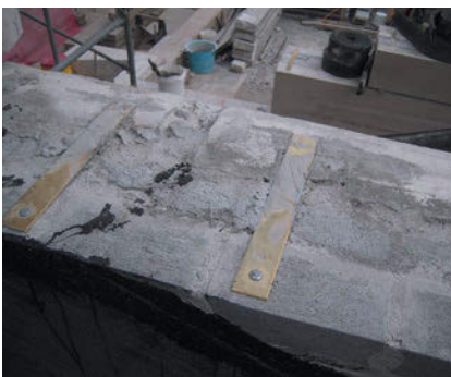
Figure 6. Stone arch reconstruction in progress at the Nebraska State Capitol. Stone grain orientation was normal to the compressive stresses within the voussoirs.
