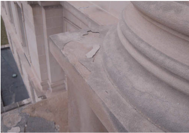
Figure 4. Spalled limestone fragments attributed to sealer applications that had previously been installed on the limestone.
