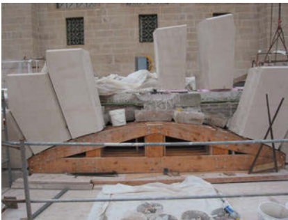
Figure 5. Reconstructed mass masonry walls with Indiana limestone and aged concrete brick back-up masonry.
