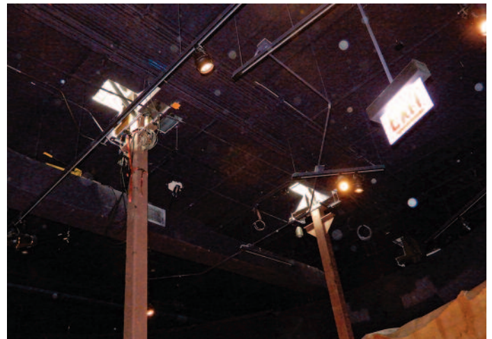
Figure 5. View from below of two of the three supplemental columns installed below the SUE gallery.
