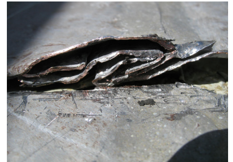
When cut open, it was found that the solder was not sweat through at all. All of the layers (four typically, but six in the photo due to the presence of a cleat) should be completely filled with solder.
