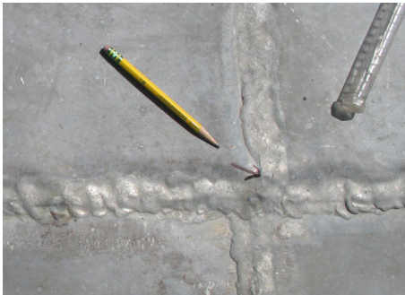
Contrary to industry standards, the locked and soldered seams in this flat seam lead-coated copper roof were soldered using a torch rather than an iron.
