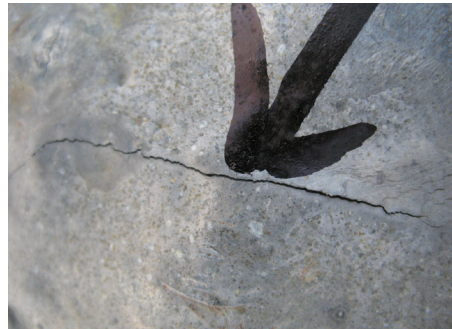
Many of the seams cracked.
