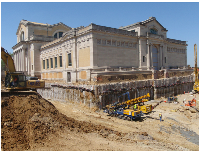
Figure 2: Earth retention system and deep excavation for expansion to The Saint Louis Art Museum, with active art galleries inside museum walls
