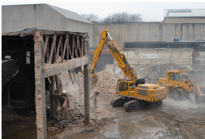
Figure 1: Demolition of existing buildings and buried seawall adjacent to active art galleries at The Art Institute of Chicago
