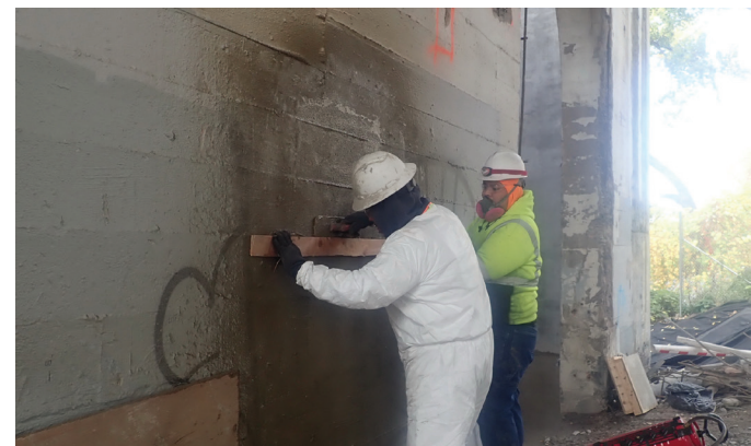
Fig. 8: Example of board-form finish achieved using hand floats in shotcrete surface repair (photograph by WJE).
