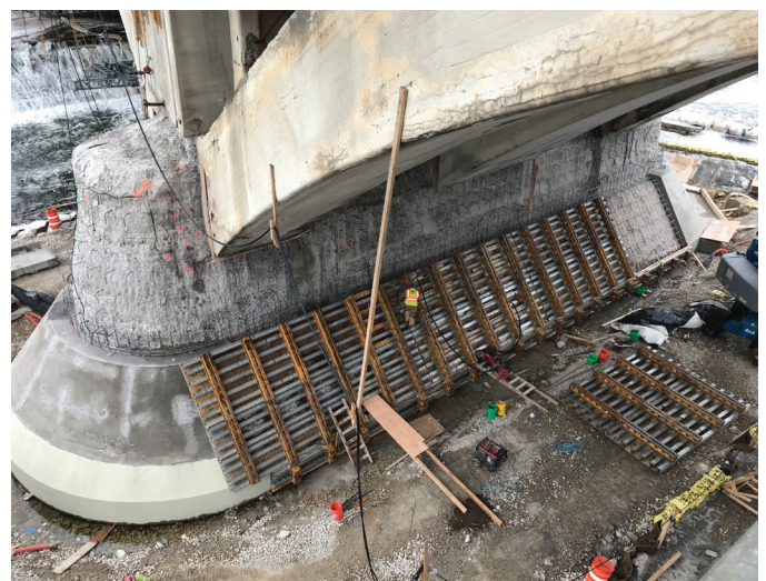
Fig. 5: Concrete removals completed, reinforcing steel being placed, and new pier jacket concrete being formed and placed (photograph by WJE)
