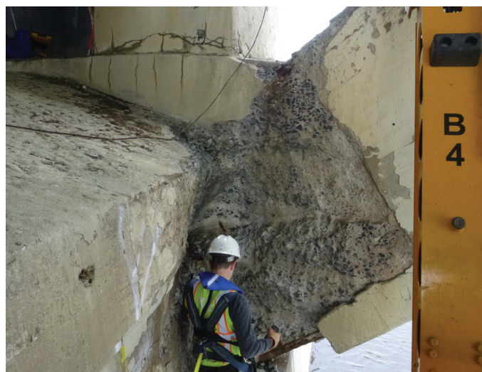
Fig. 4: Deep freeze-thaw deterioration near springline of arch rib below drain discharge (photograph by WJE)
