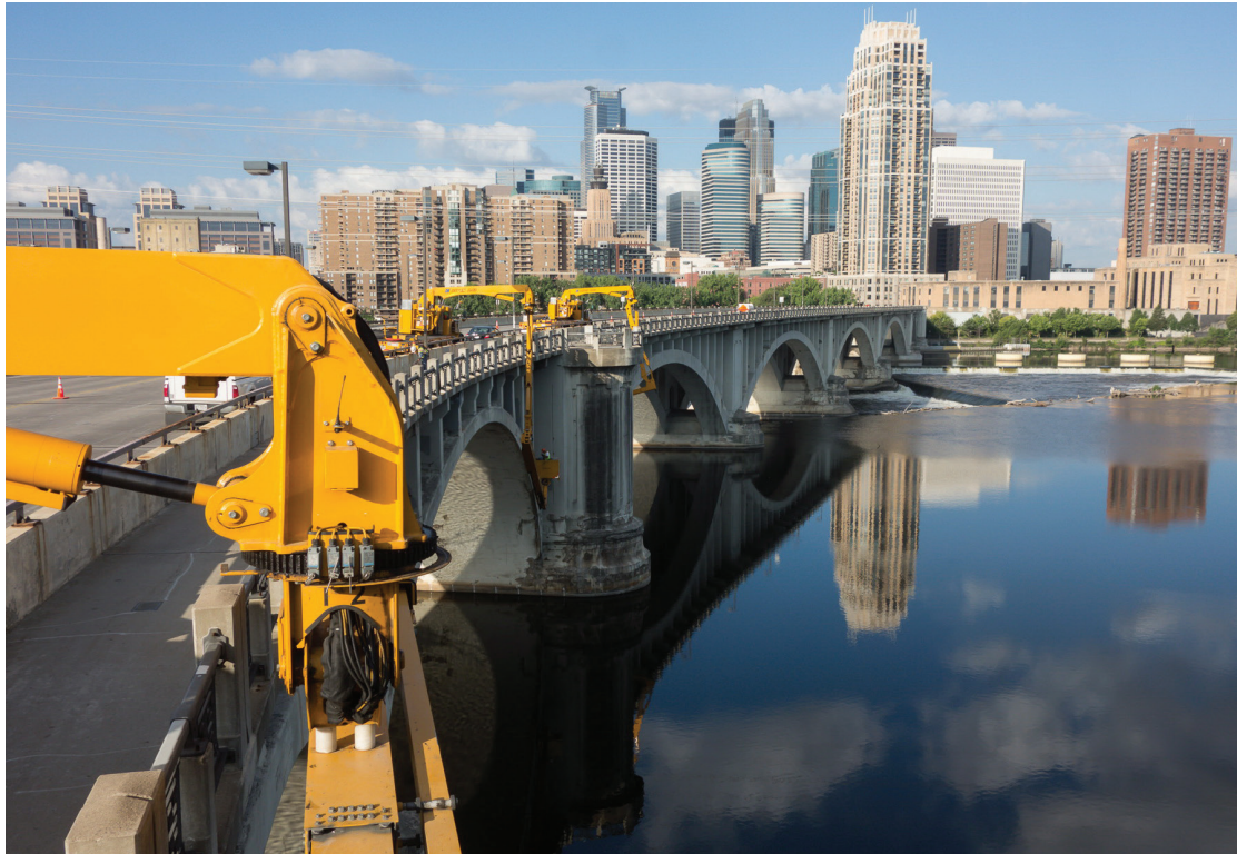
Fig. 1: Engineers utilizing three under bridge inspection units for close-up bridge inspection and sounding during the Phase 1 bridge inspection (photograph by WJE).
