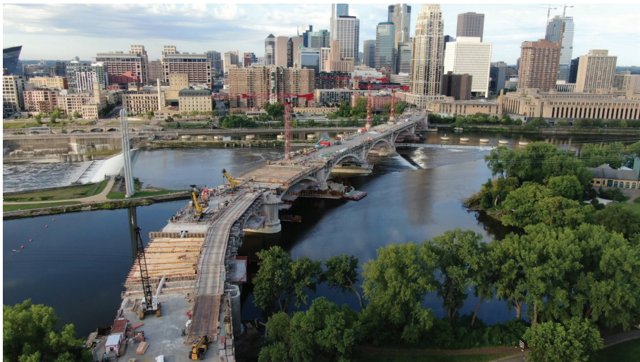
Fig. 9: Recent drone image showing status of the in-progress construction (photograph by WJE)
