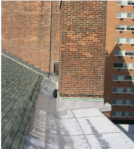
Flat seam lead-coated copper gutter comprised of very large pans and suffering from fatigue cracks.
