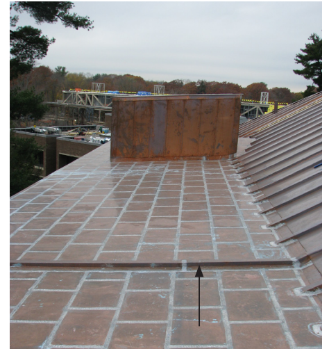
Flat seam copper roof comprised of pans no larger than 18"x24". Note also the expansion batten.
