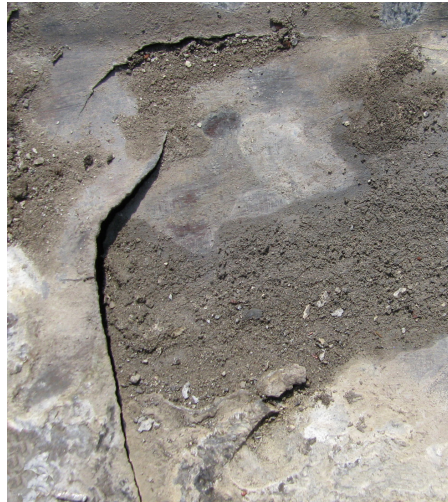
Fatigue cracks in a flat seam gutter formed from large pans with no expansion joints.
