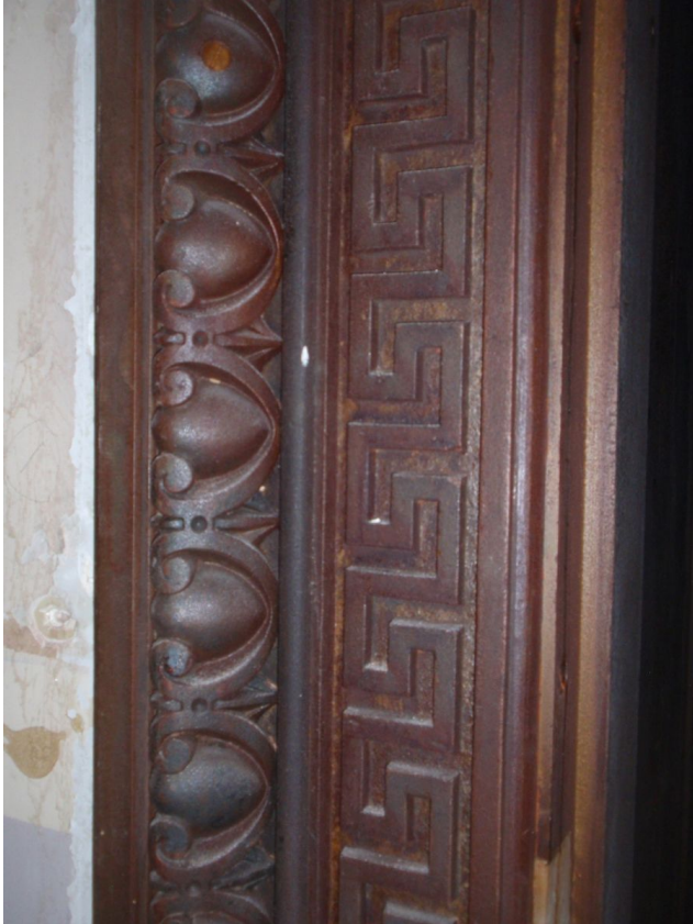
On this cast iron door trim, shown after the removal of paint using a chemical stripper, flash rust occurred during paint removal. As a result, additional surface preparation may be necessary prior to the application of new paint.
