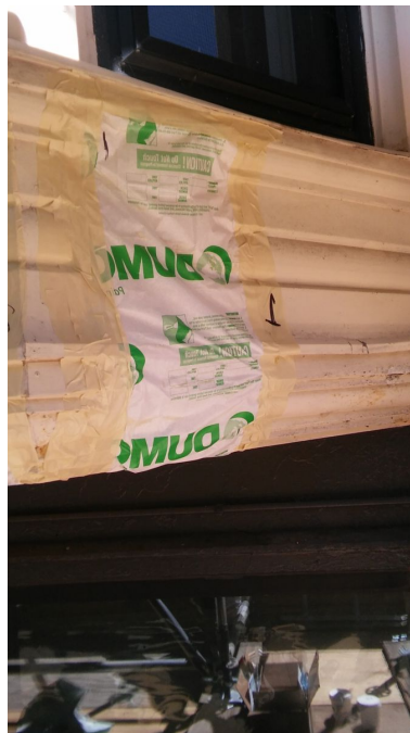
When using a chemical stripper to remove lead paint, as shown here, it is important to conduct a trial to determine which stripper is most effective, the number of applications required and the duration of each application to have the most effective results. PHOTOS COURTESY OF WISS, JANNEY, ELSTNER ASSOCIATES UNLESS OTHERWISE INDICATED
