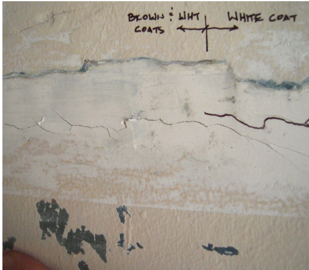
N-7. New cracks in patch at east wall observed after two months, with no changes in floor loading.
