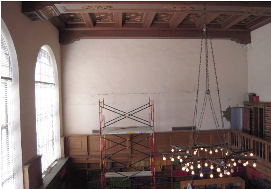
Nebraska State Library Figures N-1 top, and N-2 bottom. Historic photo from Capitol archives (left) looking west, and view of plaster distress conditions at library wall.
