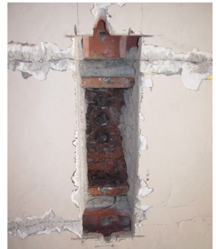
N-6. Inspection opening at east wall of Reading Room. Note the underlying concrete-encased steel beam and terra cotta tile walls above and below.
