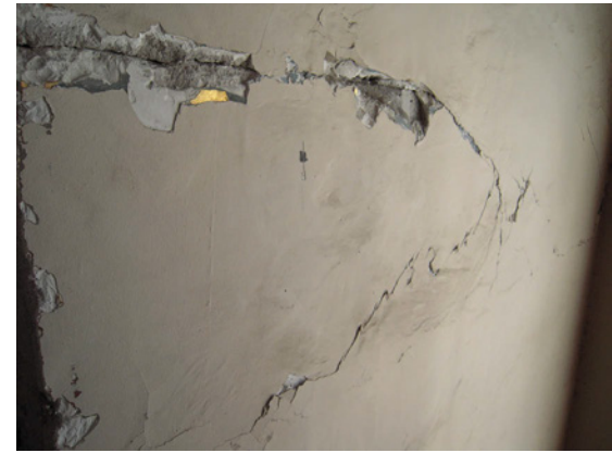
N-5. Closer view of cracks on east wall of reading room toward the south (left). Note how the cracks parallel to the top and bottom edges of the encased beam converge to a single crack near the corner of the room. View of similar cracking on west wall of room (right).
