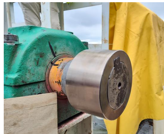
Figure 7: Custom coupling sleeve slid over the shaft, indicating the new coupling hub may be installed.
