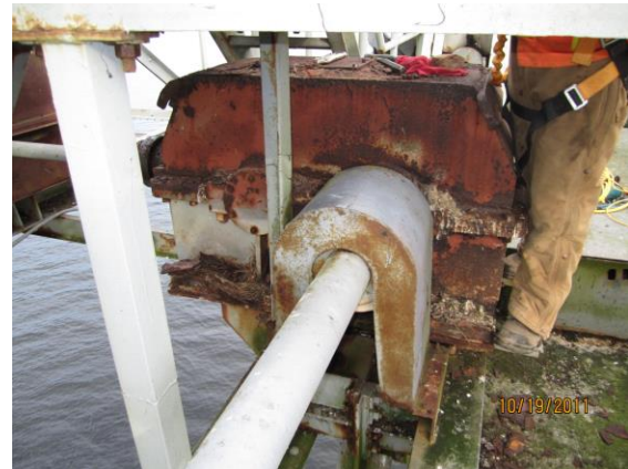
Figure 10 (above): Photograph showing coupling obscured by its protective cover.
