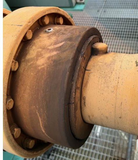
Figure 1: Coupling immediately after failure. Note fretting on exterior of the coupling sleeve, indicating internal corrosion of the coupling.
