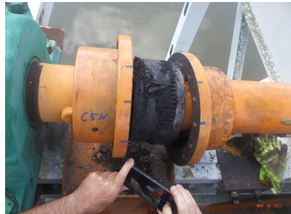
Figure 5: Coupling immediately after disassembly. Note hardened grease covering gear teeth.
