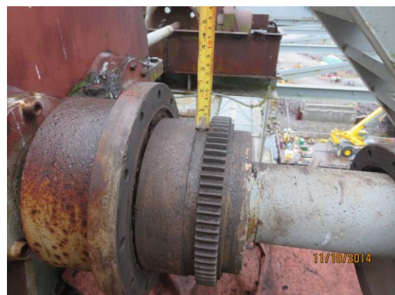
Figure 11: Photograph showing coupling with corrosive damage to be replaced.
