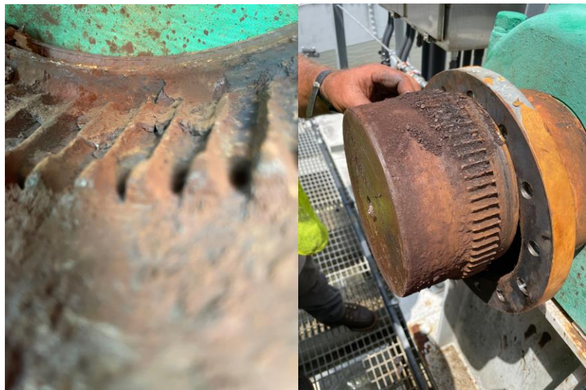
Figure 2 (Left, Sleeve) and 3 (Right, Hub): Inspection of the failed coupling. Note lack of grease, excessive corrosion and wear present.
