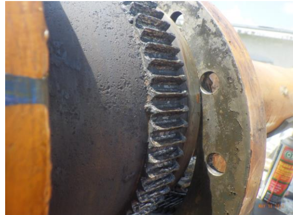
Figure 6: Coupling shown in Figure 5, after grease debris was removed. Note heavily worn and degraded gear teeth.
