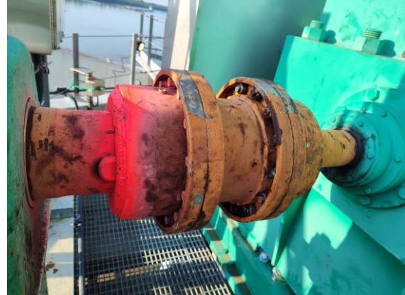
Figure 4: Weld was placed at the hub-sleeve interface of the failed coupling, marked in pink.
